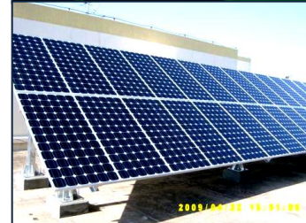
Kimhae Jinyoung water treatment center 25 kW
