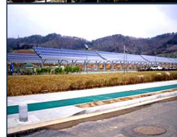
N Provincial Office (100kW)
