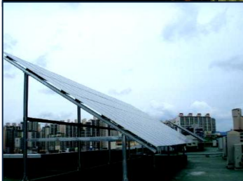
Ulsan Su Am Elementary School 30kW
