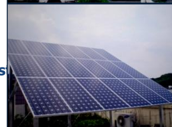
PV Home System - Chongnam 3kW
